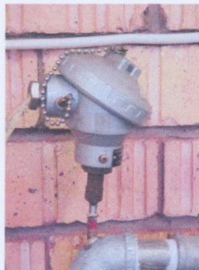
Figure 3.14 Pt100 temperature sensor with the transmitter
