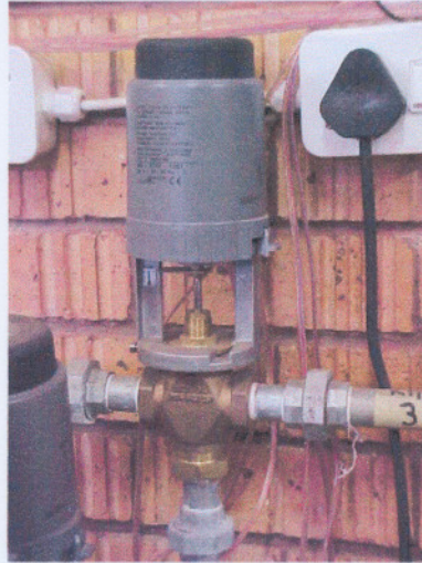
Figure 3.10 Johnson Controls VG7822LT mixing valve.
