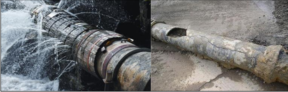
Figure 20: Pipe damage caused by water hammer 14
