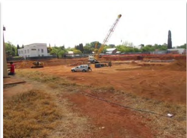
Figure 6.13 – Northern edge of the Piet Malan property, showing the depth of soil removed for the basement parking of the new apartment complex (Source: Participant 6, 2013).
