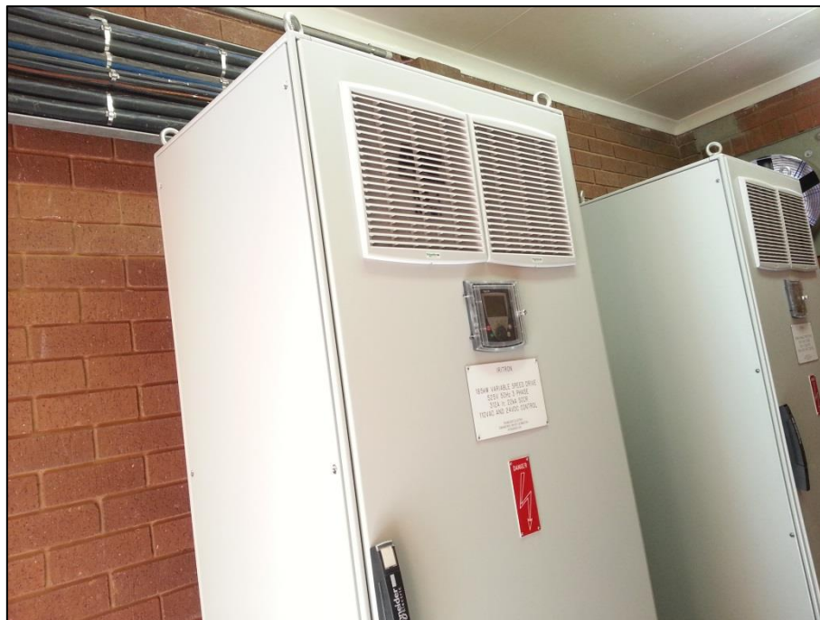
Figure 47: VSDs installed on Pamodzi evaporator pumps
