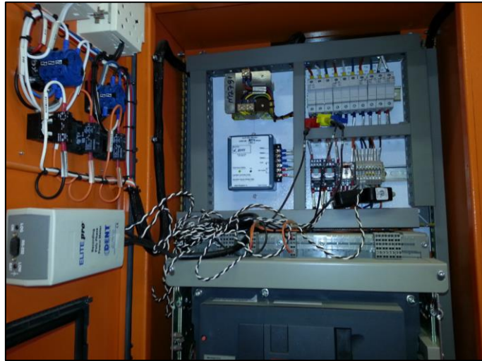
Figure 65: Installed DENT power logger
