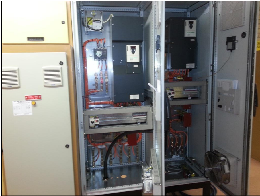
Figure 45: Inside of the York condenser (left) and evaporator (right) VSD
