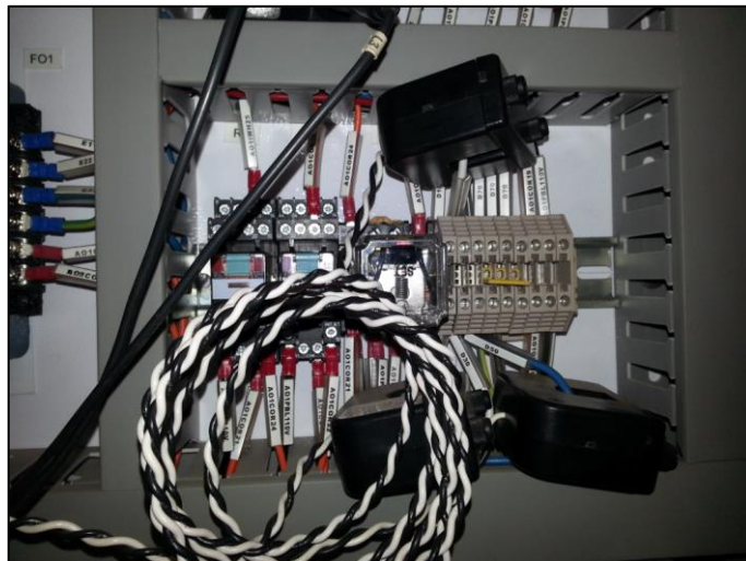
Figure 66: Current clips of DENT logger installed
