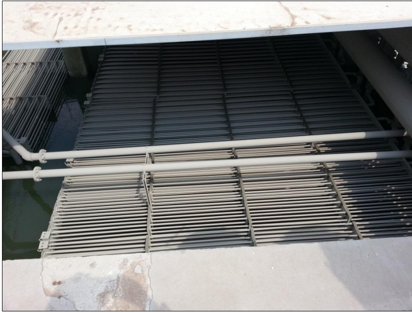
Figure 19: Tubes where ice is formed in the ice storage dam.
