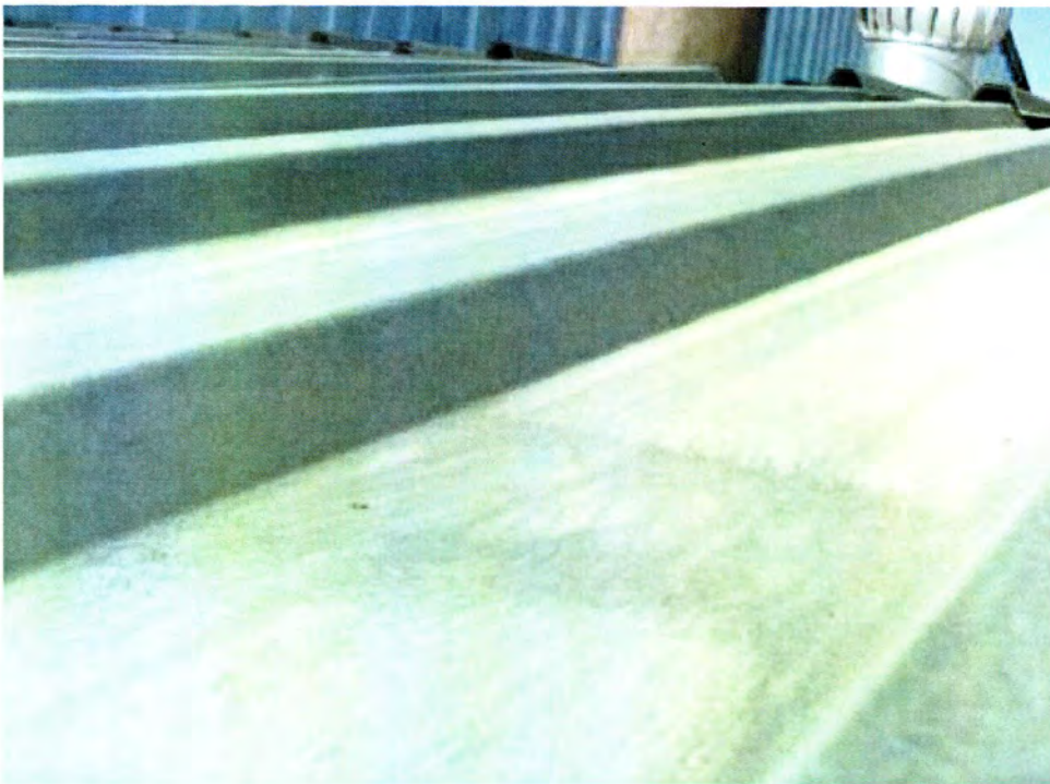
Loose dust on the kraal roof.
