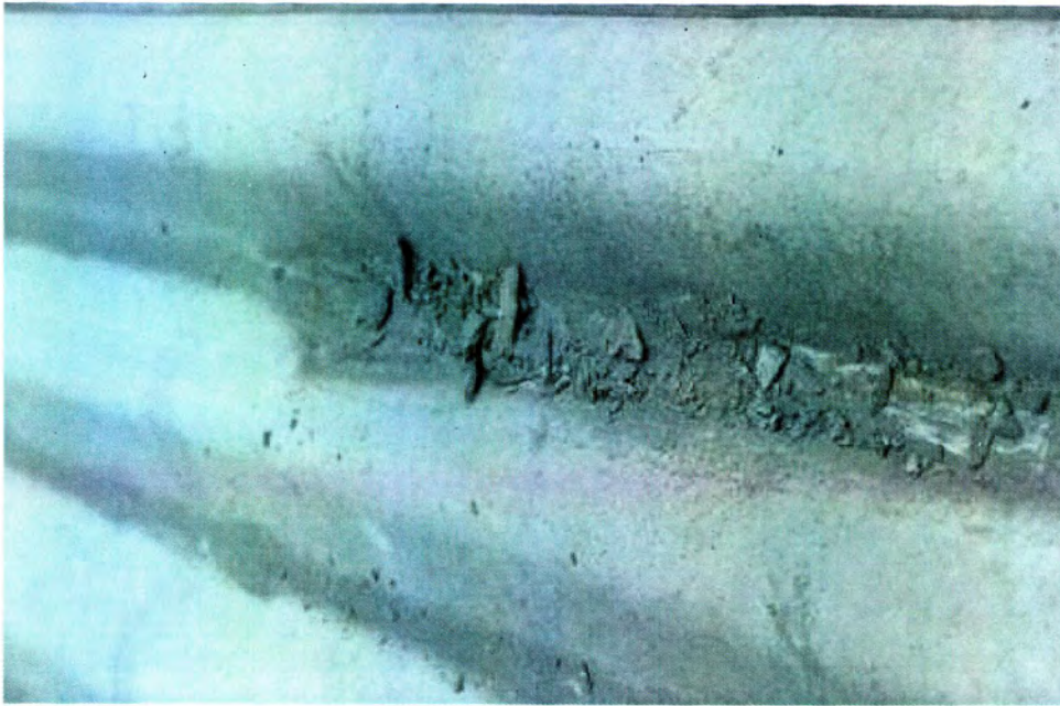
Loosened compacted dust on industrial roof.
