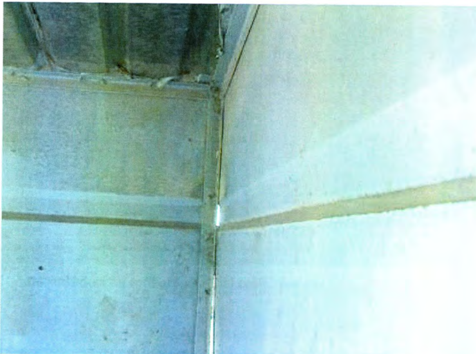
Inside panel of bus stop showing dust accumulation and compaction.
