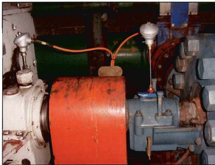
Figure 2-12: RTD probes measuring the bearing temperature and vibration on the shaft
