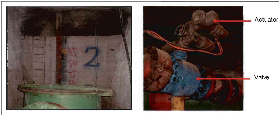
Figure 2-11: Old dam level indicator and actuated control valve (Masimong 4#)
