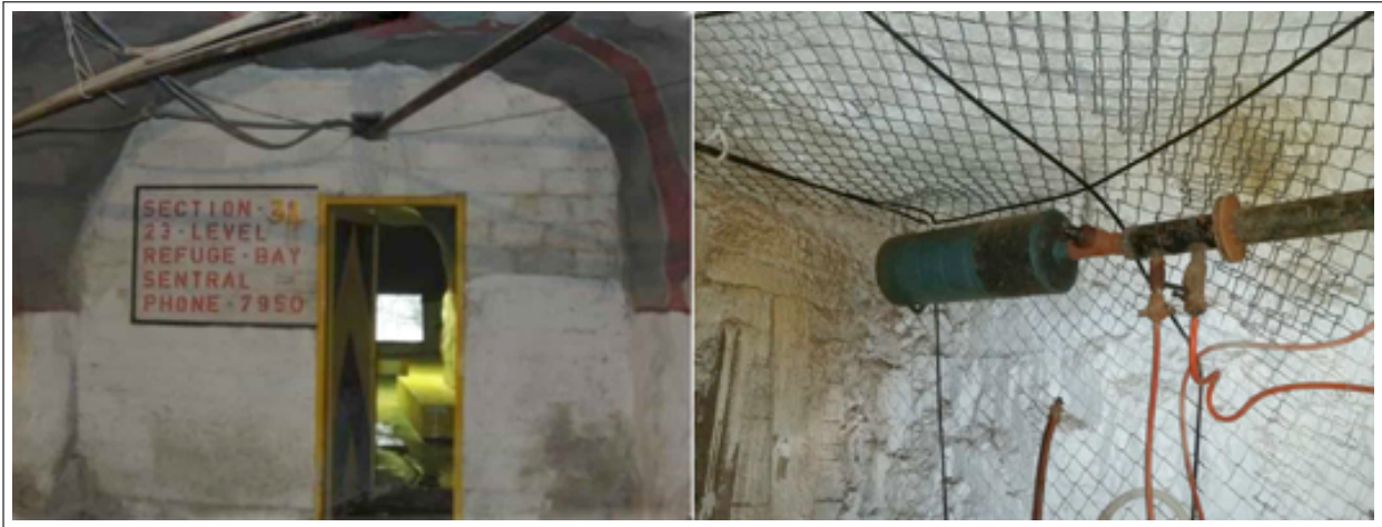
Figure 2.2: Example of a compressed air inlet in an underground refuge bay chamber of a mine
