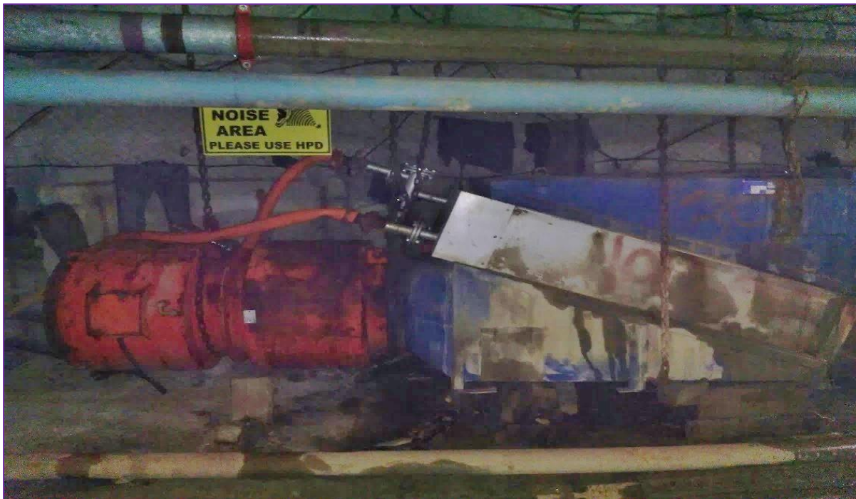
Figure 1-6: Inefficient Mobile Cooling Unit installed underground 3
