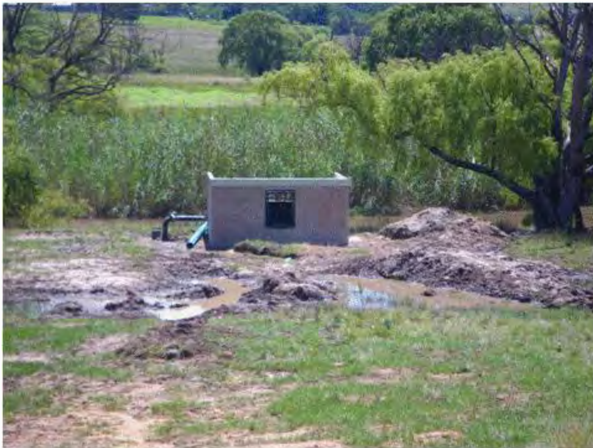
Illustration 4 Irrigation pump station along the Liebenbergsvlei River. Photograph: Martin Ginster 2009.01 31
