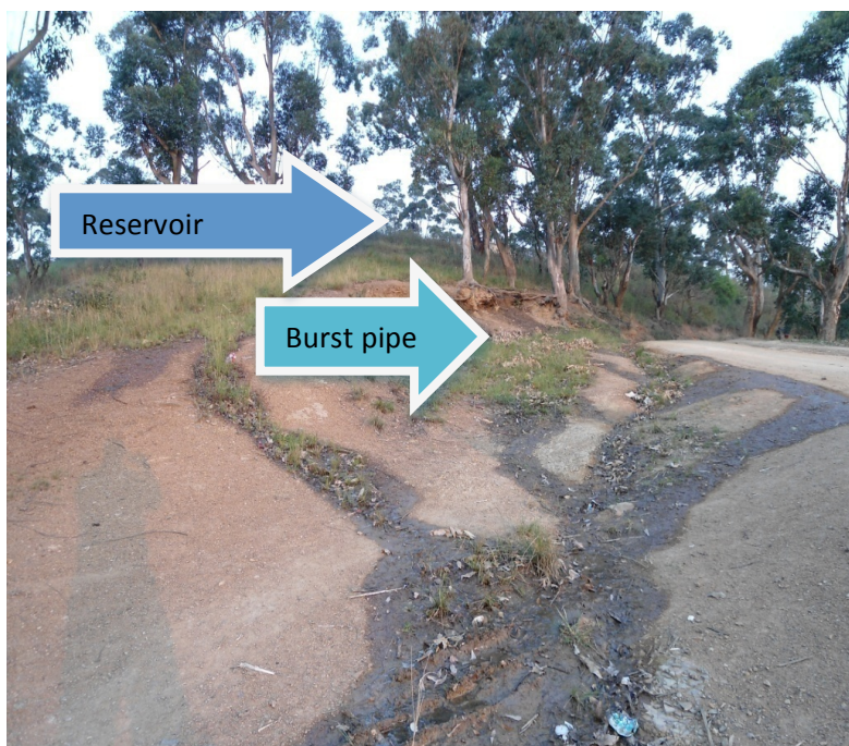
Illustration 8: Water leaking from a burst water pipe, Ward 23 Hibiscus Coast Municipality. Photographer: T. Cele
