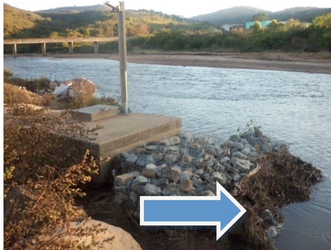
Illustration 9: Rubble covering the suction point of the water plant. In Ward 13 in the uMzambe Local Municipality. Photographer: T. Cele
