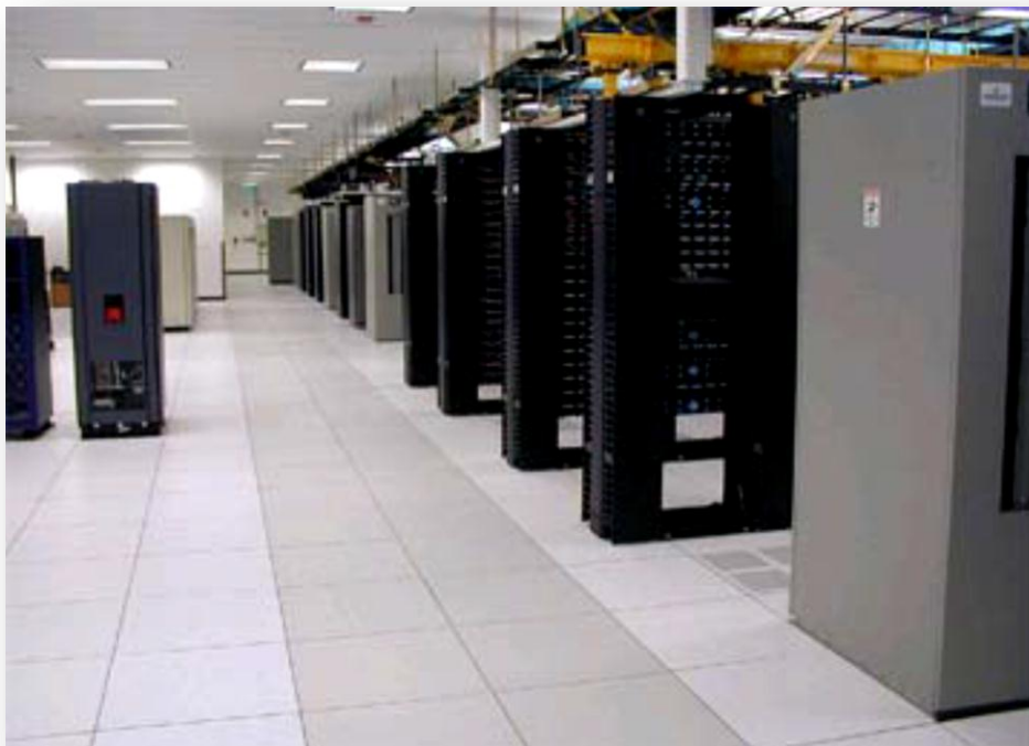
Figure 1-2: Typical data centre [16]
