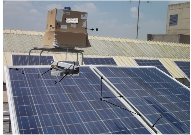
Figure 3: Water cooling system. (Outdoor setup 1 - PV module, 2 - pump, 3 - solenoid valve, 4 - sprayers, 5 - hose, 6 - water tank covered with cardboard box.
