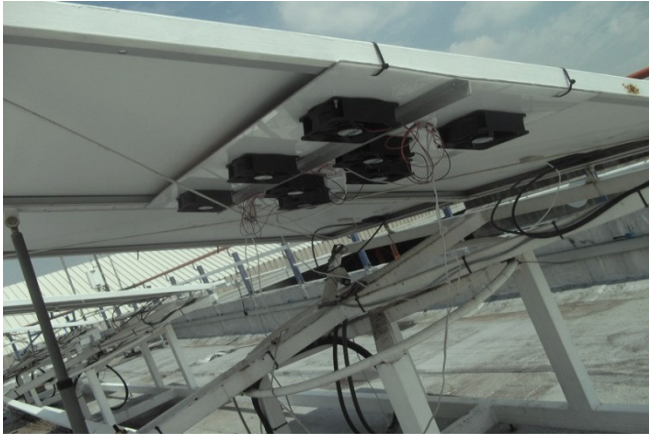
Figure 4: The back of a PV module with attached cooling fans
