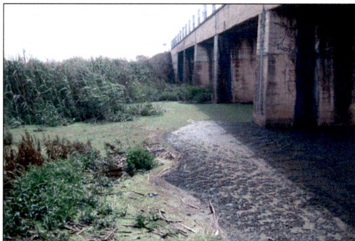
Figure 20: Evidence of raw sewage being discharged into the river
