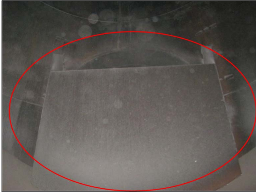
Figure 10: PA fan ducting with deflector plate
