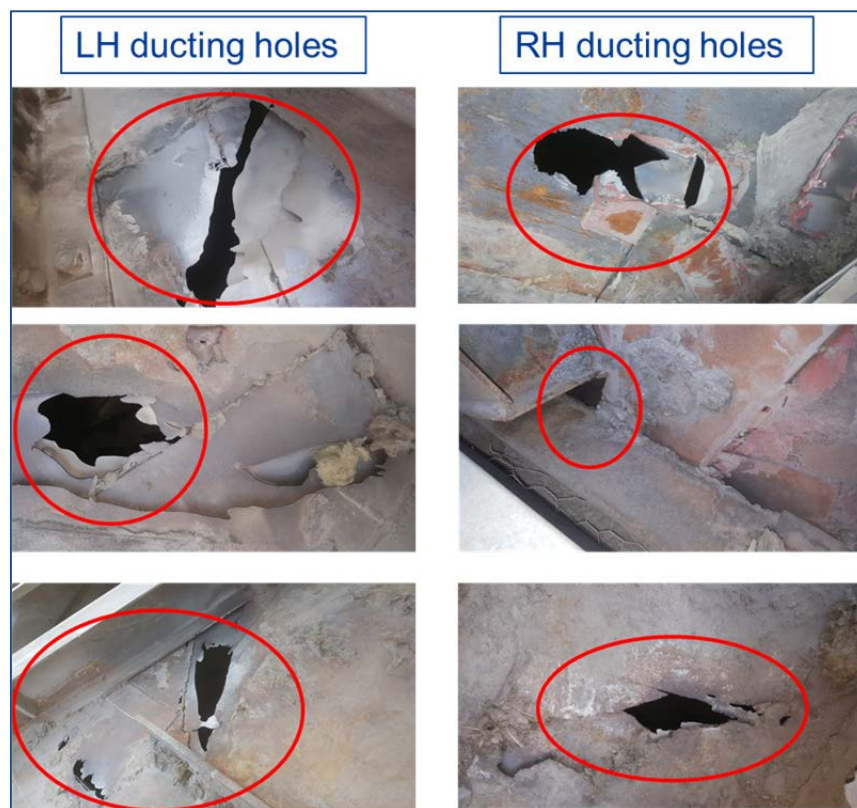
Figure 7: Power station Alpha Left Hand and Right Hand ducting holes visible after isolation removed
